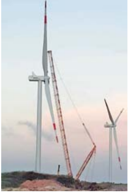
Mannar Wind Power Plant.
