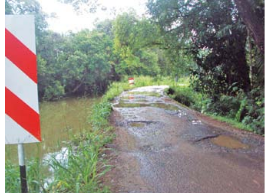
The dilapidated Pannala - Nabiriththawewa Road. Picture by Hiriyala Group Corr.
