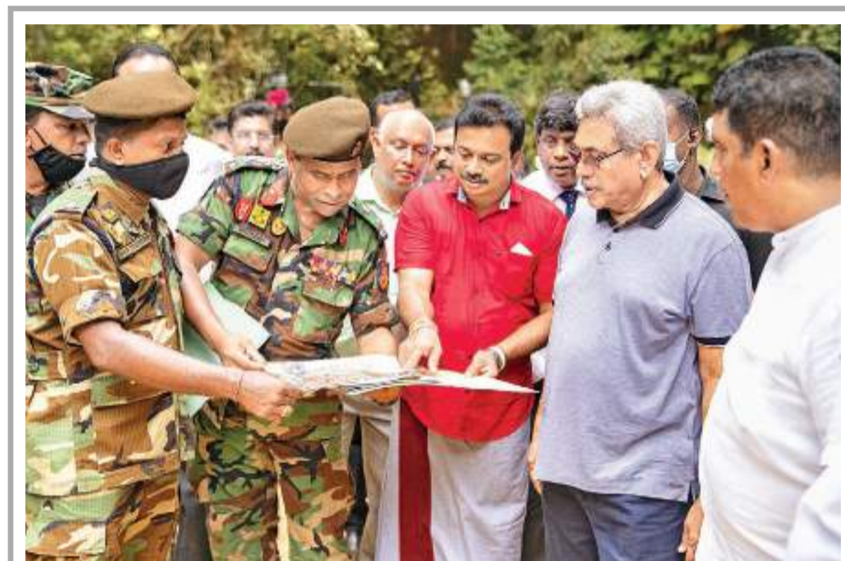
Ensuring basic needs of villagers: President Gotabaya Rajapaksa at the Neluwa-Lankagama road site where he listened to the grievances of the villagers with no road connecting their villages to main towns, directed the officials to continue the road construction work without harming the environment. He was accompanied by Highways Minister Johnston Fernando, Environment Minister Mahinda Amaraweera, Plantation Industries Minister Ramesh Pathirana, State Minister Mohan de Silva, MPs Sampath Athukorala, Nipuna Ranawaka, Chandima Weerakkody, Weerasumana Weersinghe and Southern Province Governor Willie Gamage Pic: Courtesy PMD
