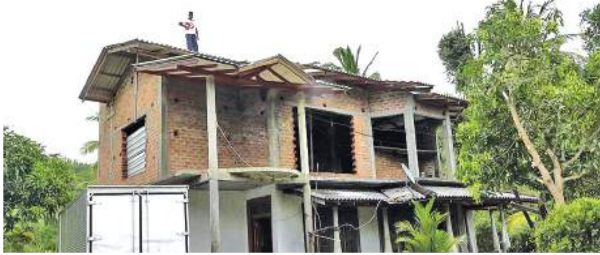
A damaged house.
