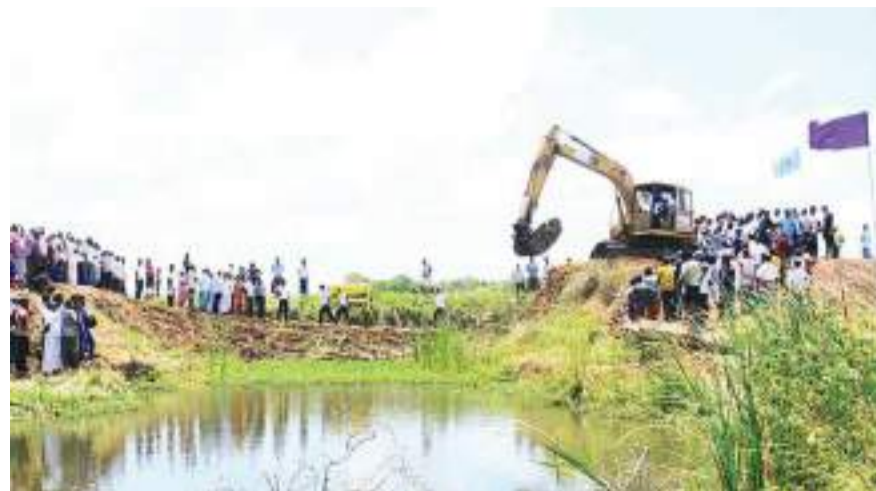
The recent inspection of the Pahala Halmillewa irrigation tank by State Minister Siripala Gamlath. The tank is to be renovated in four months.
