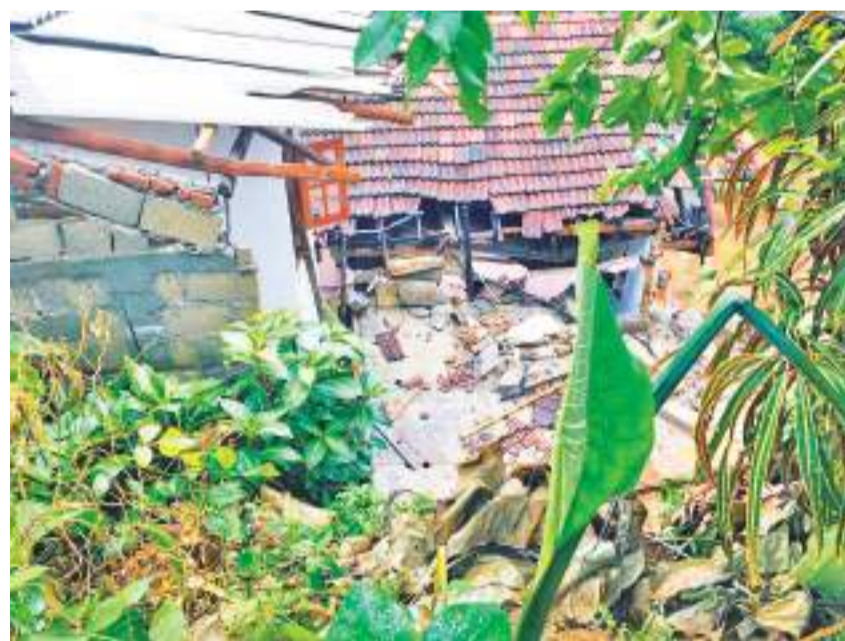
Heavy rains in the Galle District caused a parapet wall to collapse onto a house, injuring a mother and daughter in Uluwitike, yesterday. The victims have been identified as 58-year-old Kusum Rani and her 18-year-old daughter, Yasanga Madanayake. They have both been admitted to the Karapitiya Teaching Hospital for treatment.
