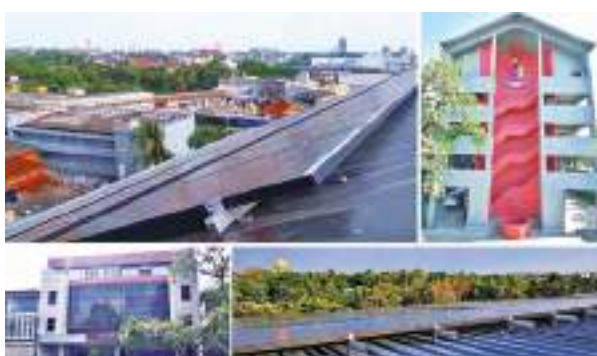
The solar panel installations at Ceylinco Life's branches in Jaffna and Anuradhapura
