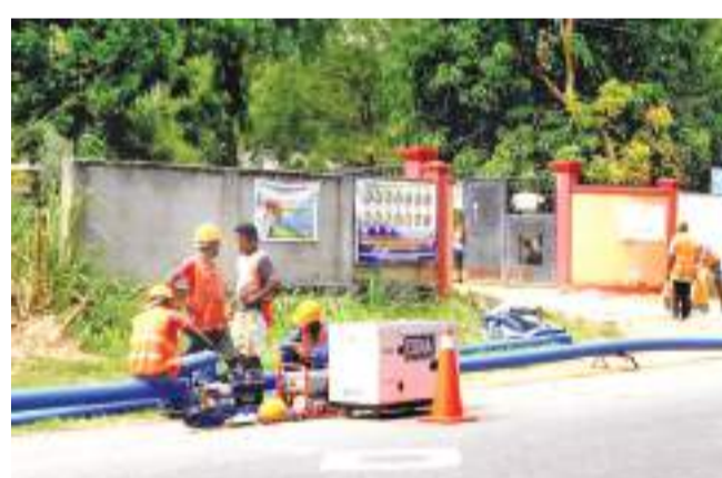
Work under the Badulla District Water Supply and Sanitation Facilities Improvement Project resumed recently after being postponed for months due to the COVID-19 pandemic. The project is being carried out on the Mahiyanganaya - Mahaoya Road. Picture by Navaratna Bandara, Mahaweli Systems Group Corr.
