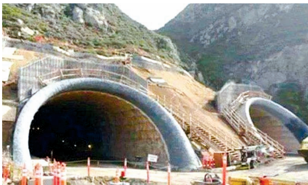
The strategic Rohtang tunnel is being built at an elevation of 10,171 ft under the Rohtang Pass in the Himalayas' eastern Pir Panjal Range.
