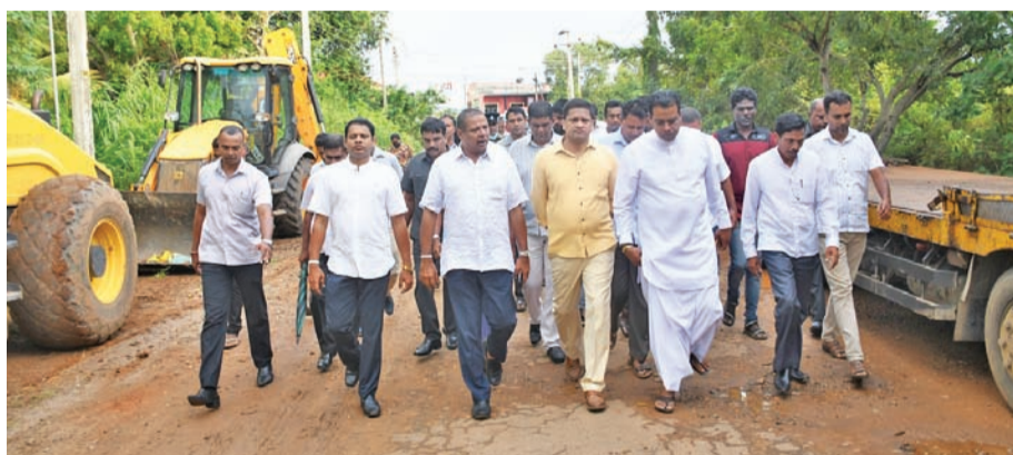
State Minister Nimal Lanza and other officials inspecting the road construction work.
