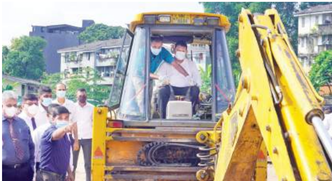
State Minister of Urban Development, Coast Conservation, Waste Disposal and Community Cleanliness Dr. Nalaka Godahewa at the inauguration ceremony to construct 400 housing units at Elliot Place Borella.
