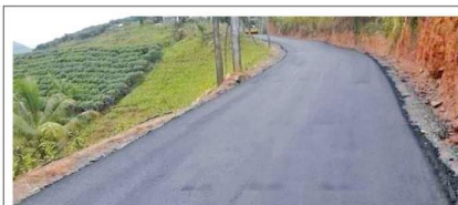
The rehabilitation of the Neluwa-Lankagama road, which has been a long-standing need for the people in the isolated village of Lankagama bordering the Sinharaja Forest range, is in its final lap. The road will be completed within 90 days under President Gotabaya Rajapaksa's directive. Picture by Raveendra Liyanage.
