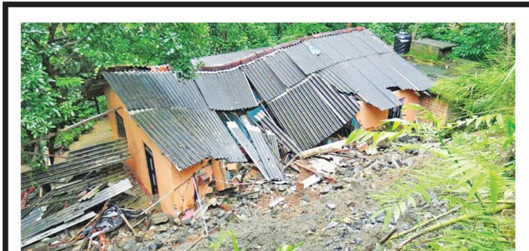
The house that collapsed in Medabedda in Galewela. Picture by Kanchana Ariyadasa.
