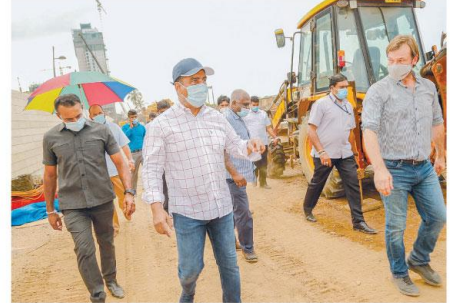
Highways Minister Johnston Fernando made an inspection tour to observe the construction work being carried out on the extension of Marine Drive
