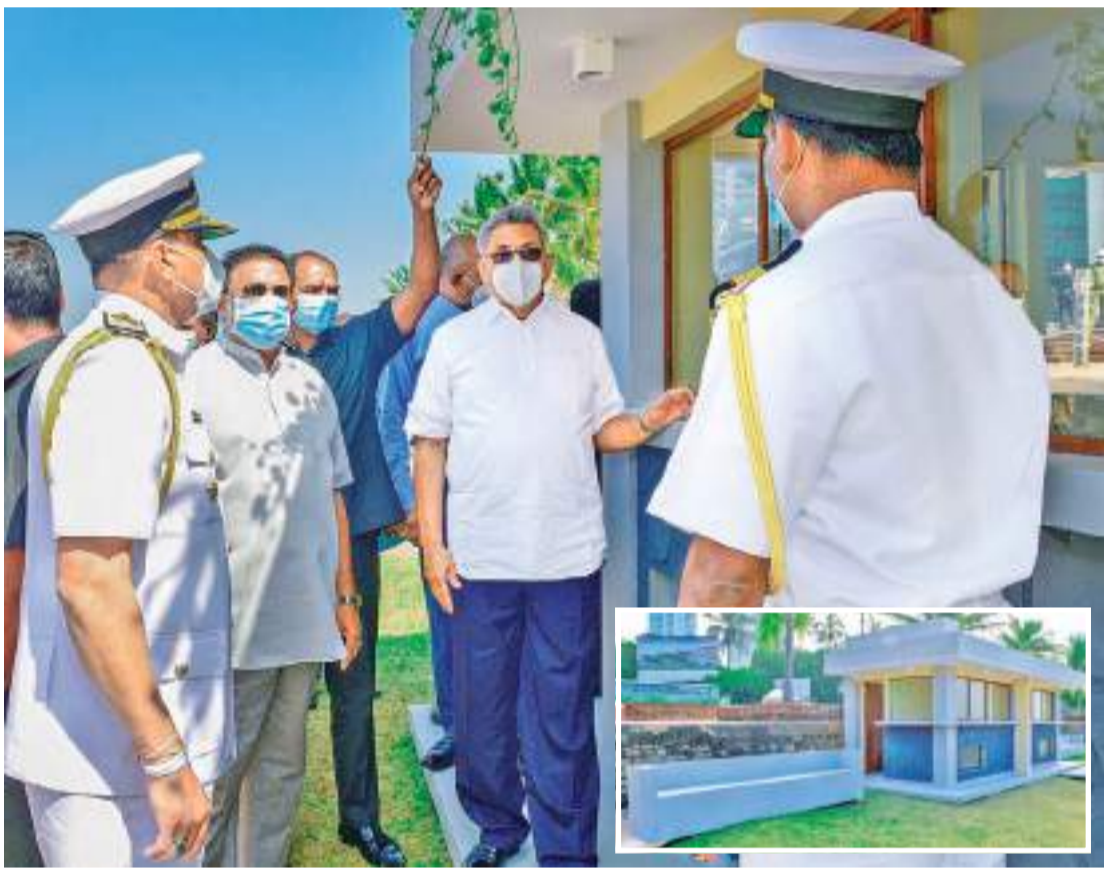
President inspects construction of model stalls at Galle Face Green in Colombo yesterday morning. The line of stalls will be constructed as another step in the development project surrounding the Galle Face Green. The Navy has designed these model stalls according to the envisioned new plan. President Rajapaksa stressed the need to build the stalls enhancing the scenic appearance of the Galle Face Green. Minister Rohitha Abegunawardhana, Navy Commander Vice Admiral Nishantha Ulugetenne, Sri Lanka Port Authority Chairman General (Retired) Daya Ratnayaka and several others were present on the occasion. Picture courtesy President's Media Division
