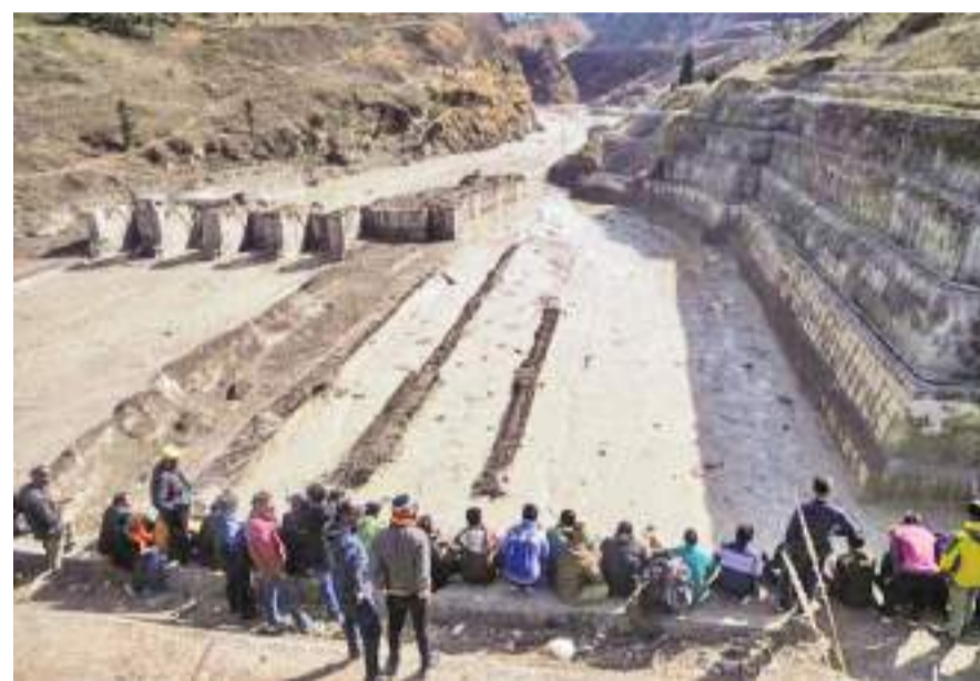
A dam along a river in Tapovan was severely damaged in the flash flood.
