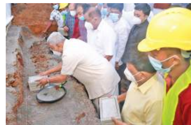
Work on three-storeyed building complex comprising an auditorium for the trade union centre 'Sevaka Piyasa' of the SLPP commenced yesterday on Nelum Mawatha, Battaramulla. Here, Minister Chamal Rajapaksa laying the foundation stone.
