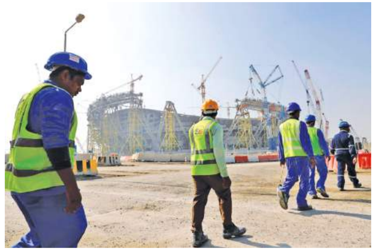
Workers at a construction site of a World Cup venue in Qatar
