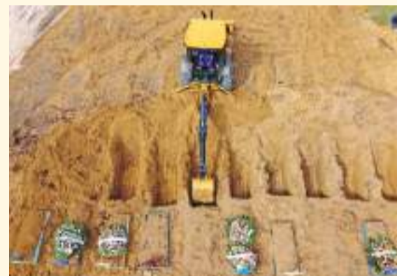
An aerial view of a tractor digging graves in a new area of the Nossa Senhora Aparecida cemetery reserved for COVID-19 victims, in Manaus, Brazil. - AFP
