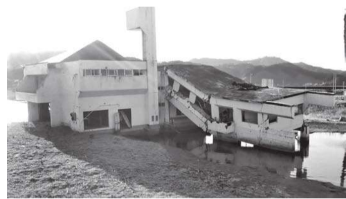
This building in Rikuzentakata has been left untouched since the disaster, in memory of the tragedy.
