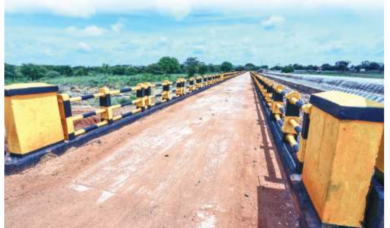
The bridge at the Vavunikulam tank. The Vavunikulam tank is an ADB-supported project with a 3.5 km bund, a bridge, and a canal as an emergency project to restore and improve the livelihoods through economic infrastructure development in the conflict-affected areas in Vavunikulam.
