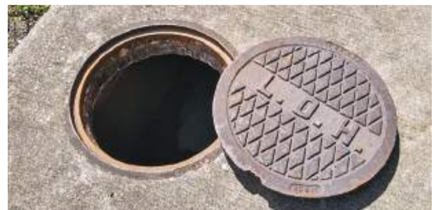
An open manhole
