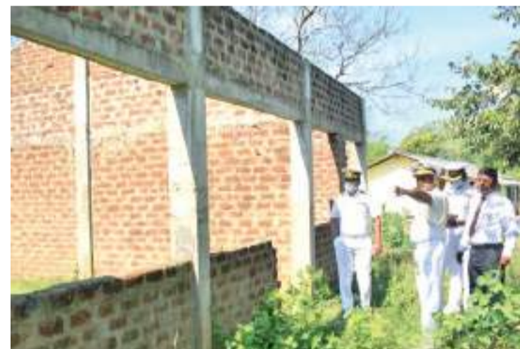
The half-completed classroom building of Pansalgodella Primary School being inspected by the Navy.
