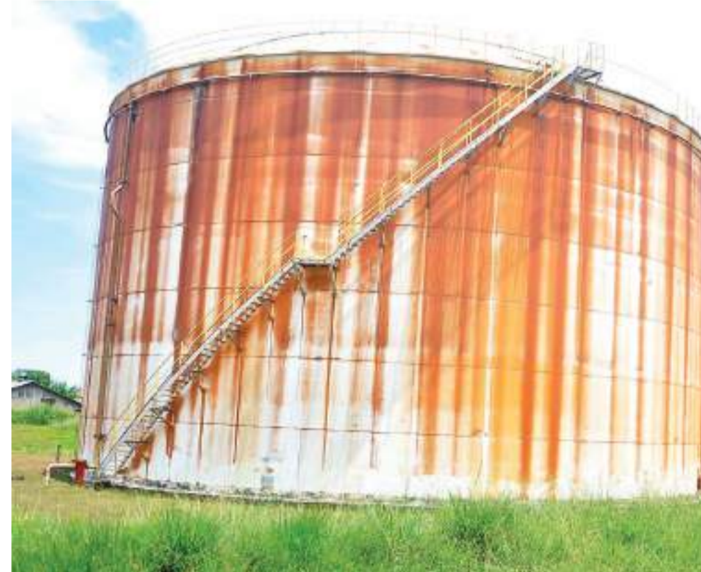
One of the oil storage tanks damaged and left to idle for over 10 years
