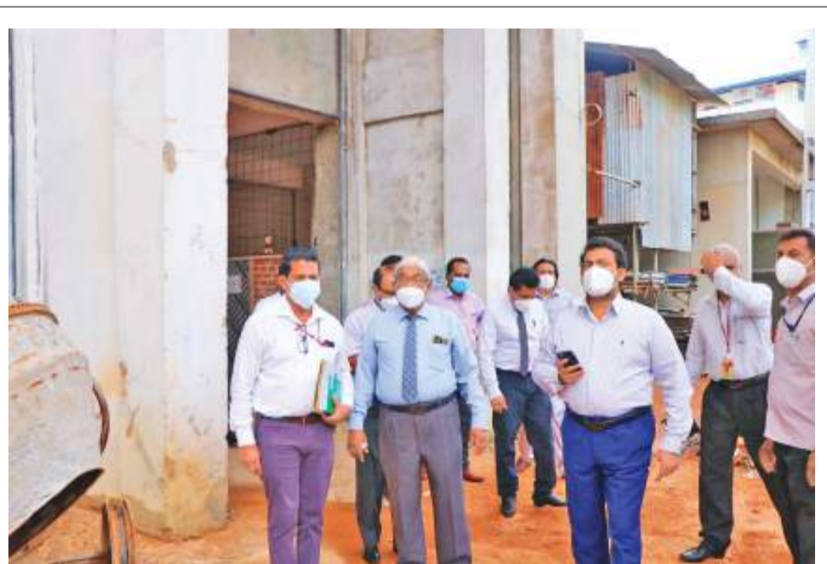
Rural Housing and Construction State Minister Indika Anuruddha inspected the work on the 10 storey building at the Colombo South Teaching Hospital Kalubowila being built at a cost of Rs. 743 million. The construction is being carried out by the State Engineering Corporation. The new building consists of seven operating theaters, five laboratories and two Outdoor Patients Departments. Picture by Ashraff A Samad
