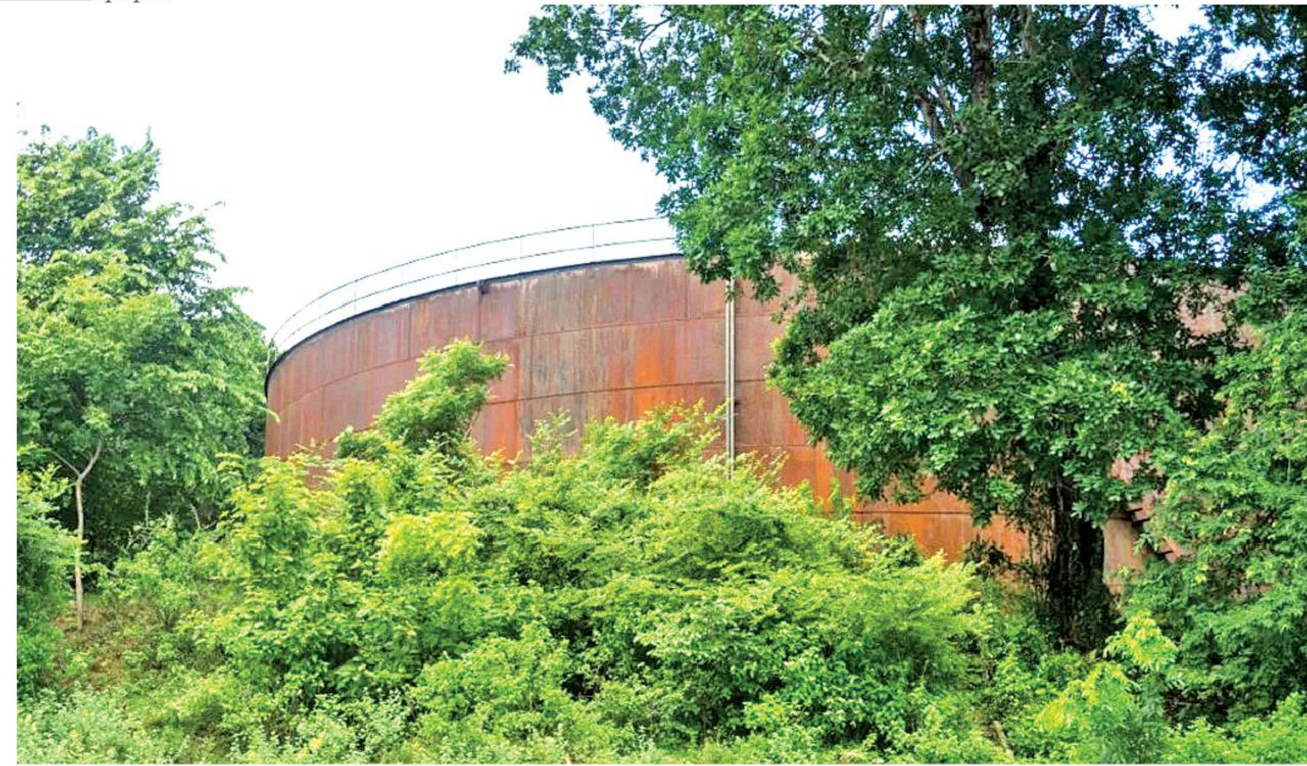
An abandoned tank at the Trincomalee Oil Storage Facility.
