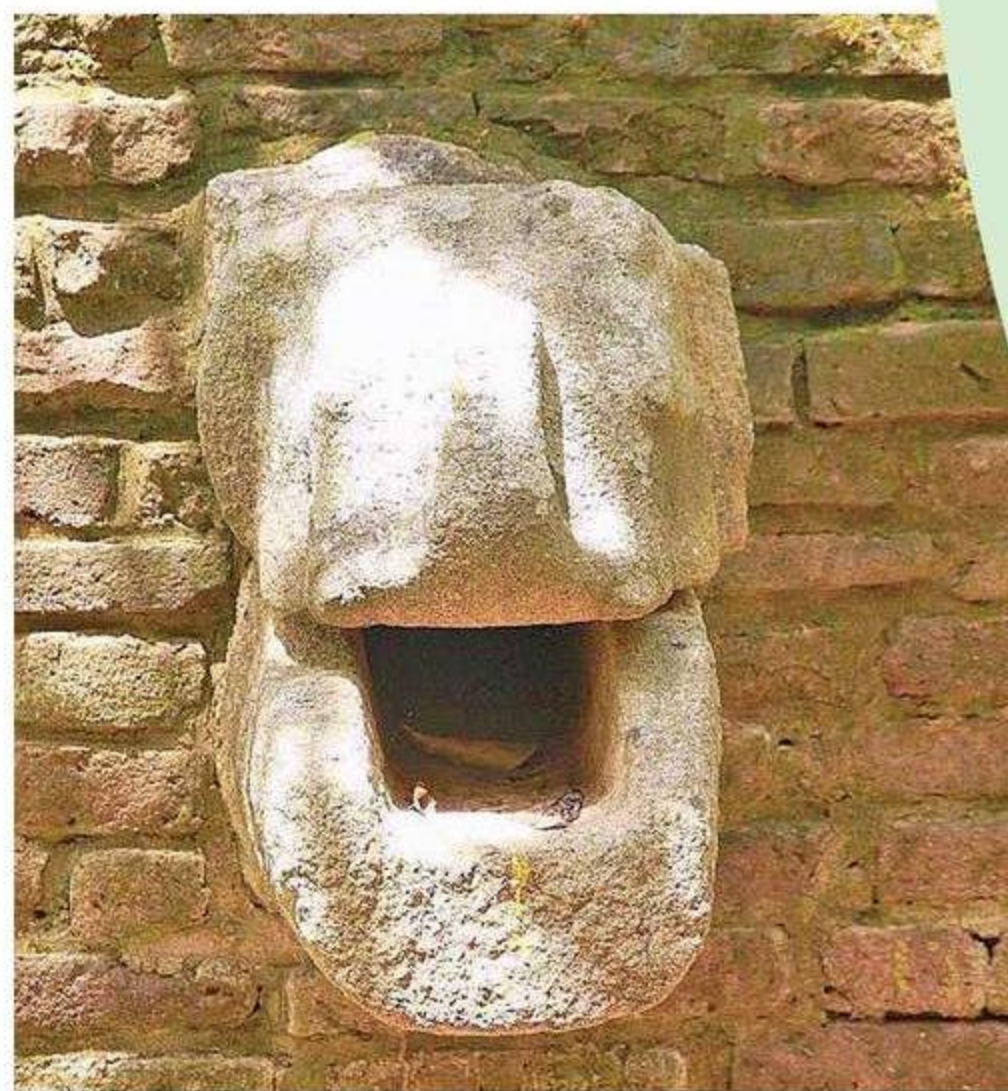
Sprouts to drain water.
