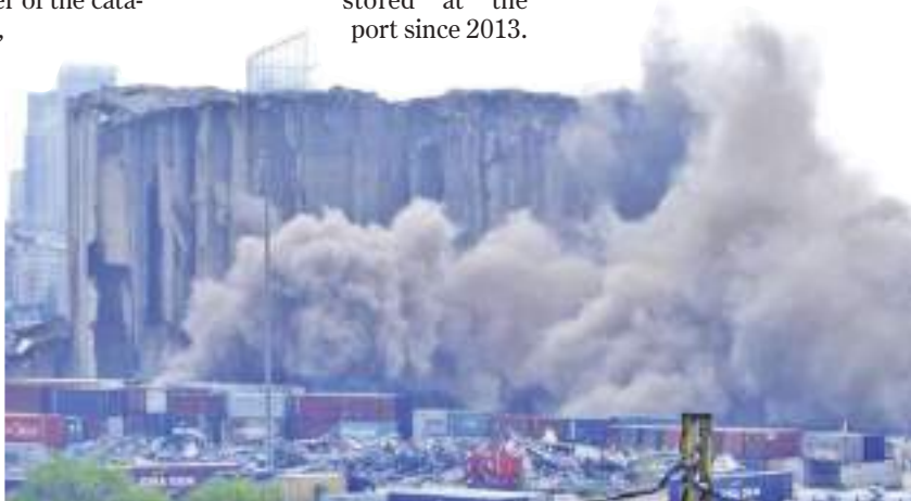
This frame grab from video shows part of the silos collapsing, in the port of Beirut, Lebanon on Sunday.
