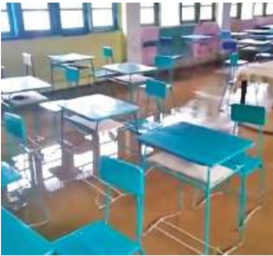
The classroom of a school in the Nuwara Eliya district flooded after heavy rains.
