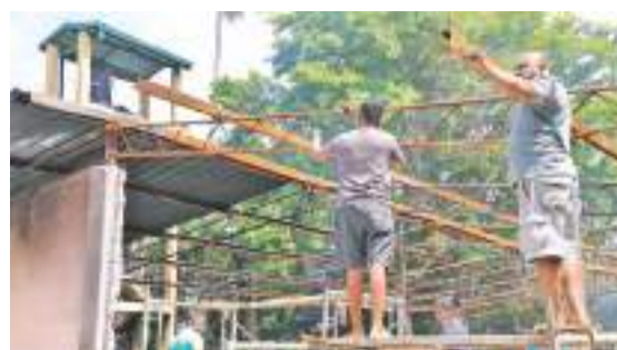
Renovation work on Minister Prasanna Ranatunga's political office being carried out by supporters and area residents.
