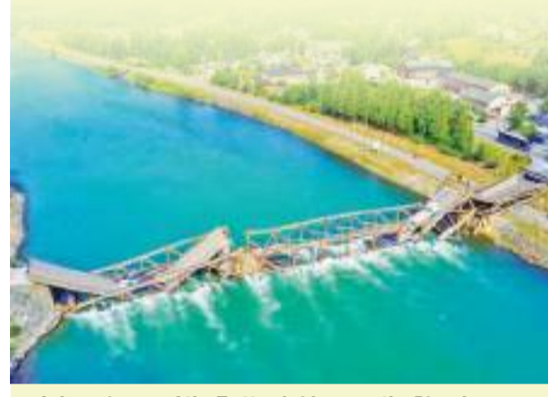
A drone image of the Tretten bridge over the River Laagen that collapsed, in Gudbrandsdalen, Norway on Monday.
