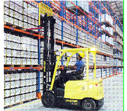
MHE racking system
